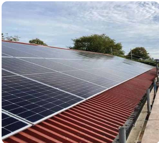
Solar PV installation at our Jubilee Toilets, installed in 2022.
